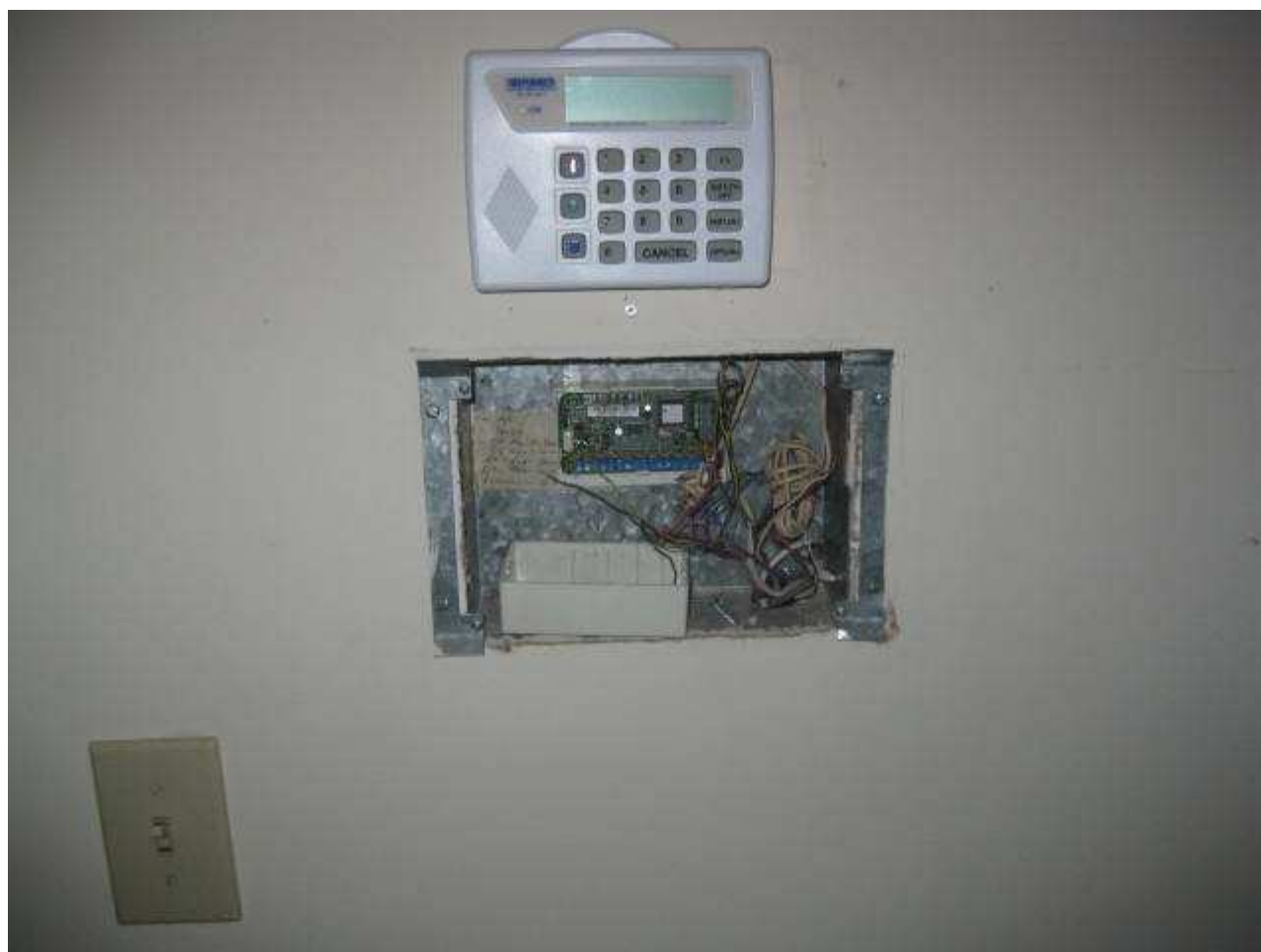
Hole in wall.JPG
